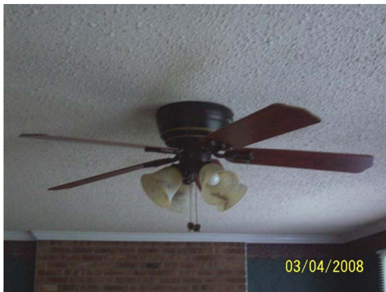
Living room ceiling fan not functional
