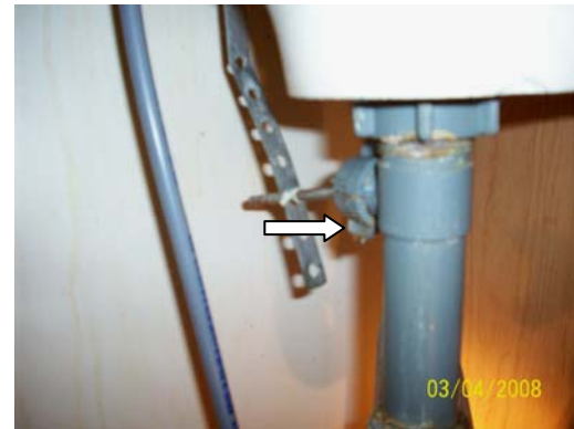
Detached garage sink basin with leaking drainage pipe
