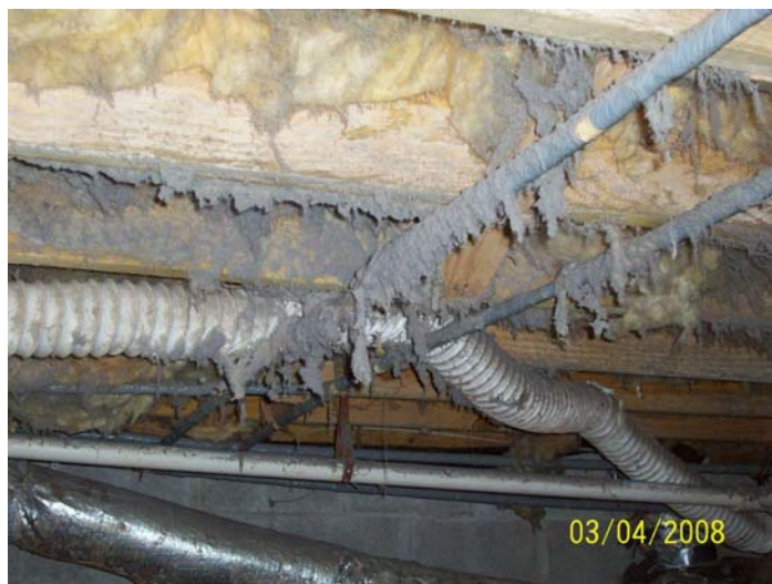
Excessive dryer lint located in crawlspace interior
