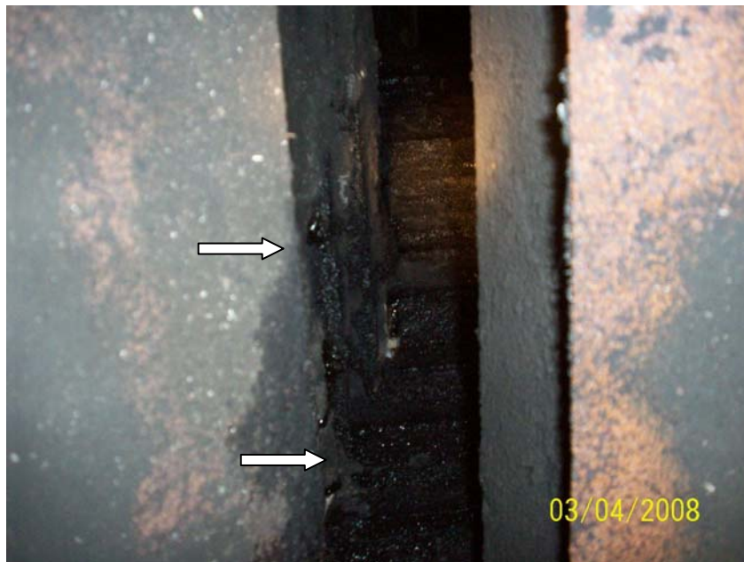
Interior chimney with water penetration located beneath the flue
