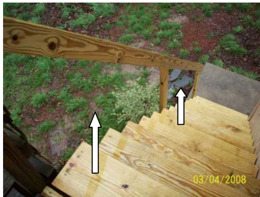
Rear wood deck stairwell hand railing with improper vertical balusters
