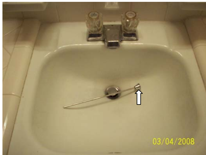
Hallway bathroom with damaged drain stopper hardware
