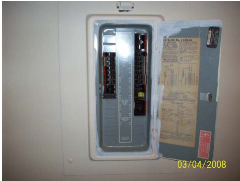
Federal pacific stab-Lok main service panel
