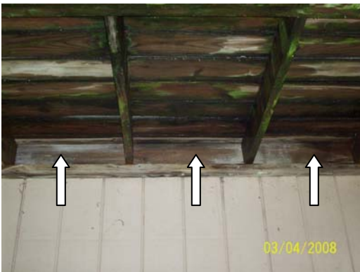
Rear wood deck with uninstalled lag screw hardware
