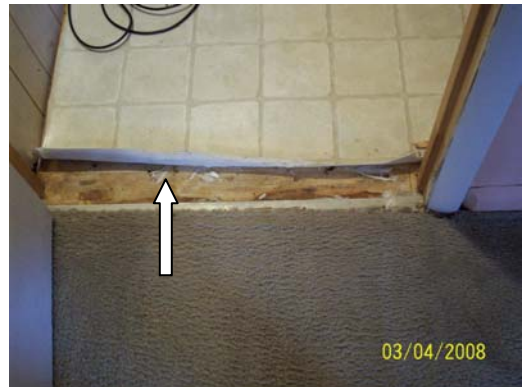
Detached garage upper level with damaged vinyl floor covering
