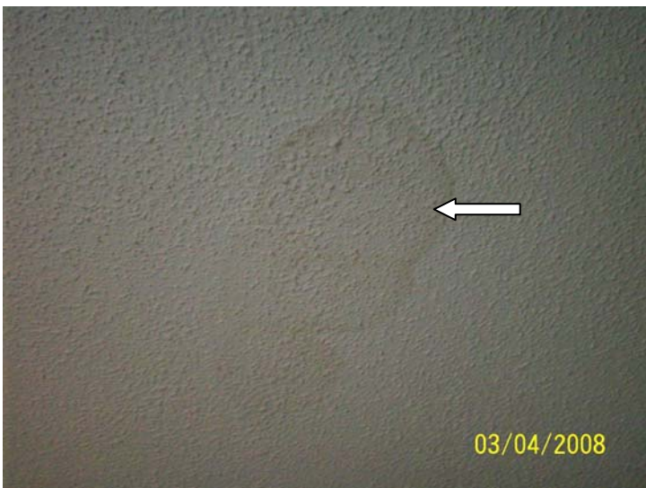
Interior family room with evidence of past or present water staining
