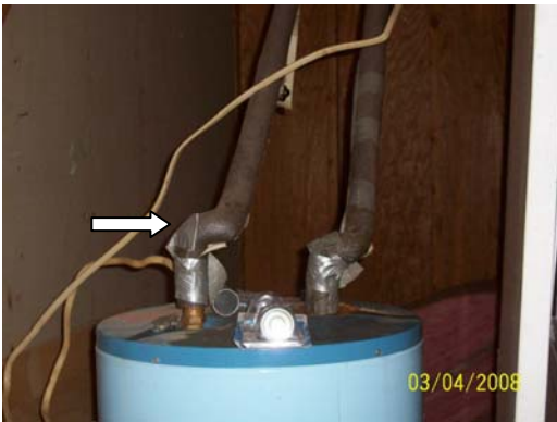
Leaking hot water supply line
