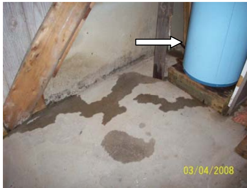
Water heating unit 13 years old
