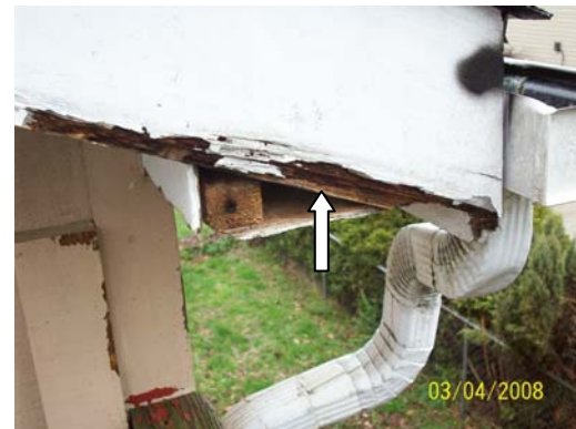
Wood fascia trim with rot and deterioration
