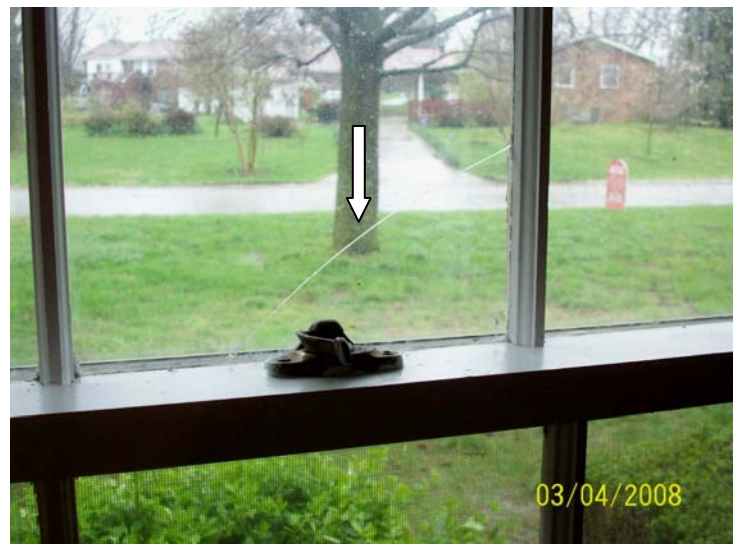
Interior living room window with glass damage
