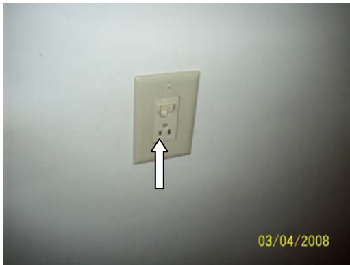
Detached garage electrical receptacle not functional
